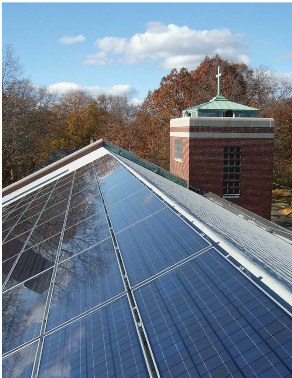
Christ Church, Teaneck, is one of several churches in the diocese to install solar panels.
